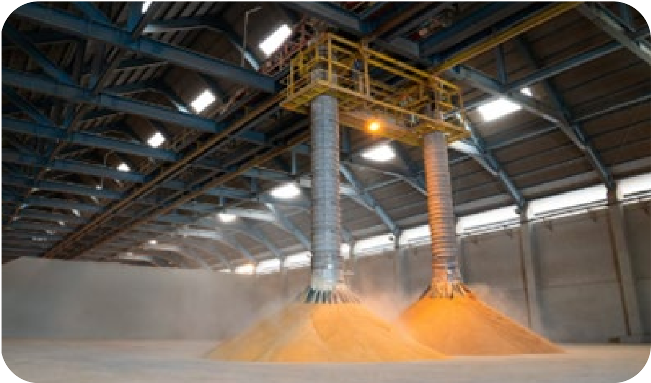
Telescopic Chute di Sentral Gudang Terminal - Medan Telescopic Chute at the Sentral Gudang Terminal - Medan
